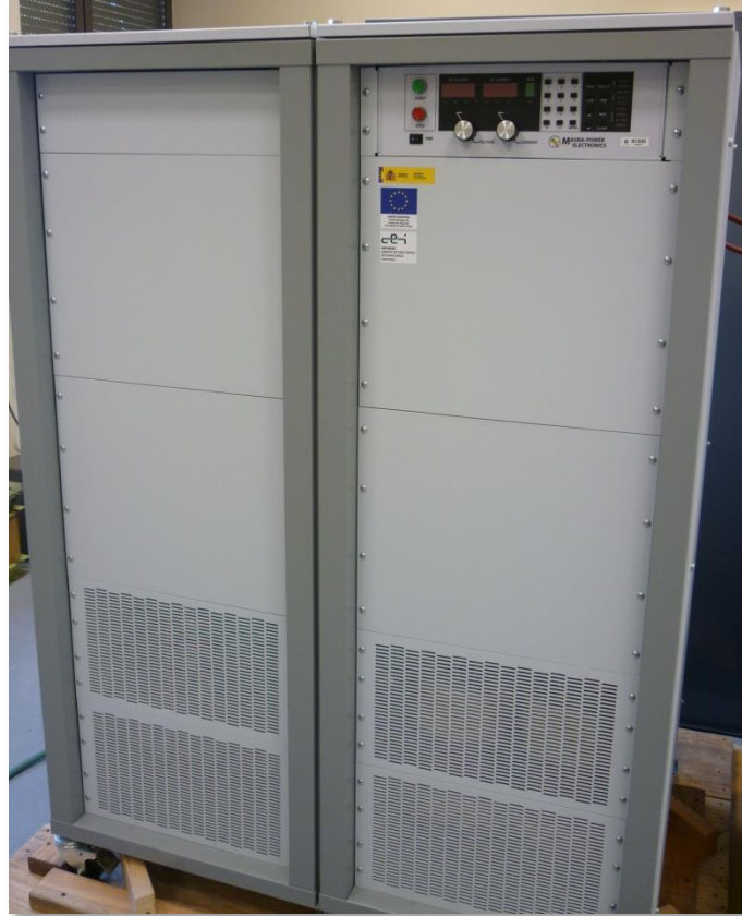
Fig. 31 DC Power Supply
