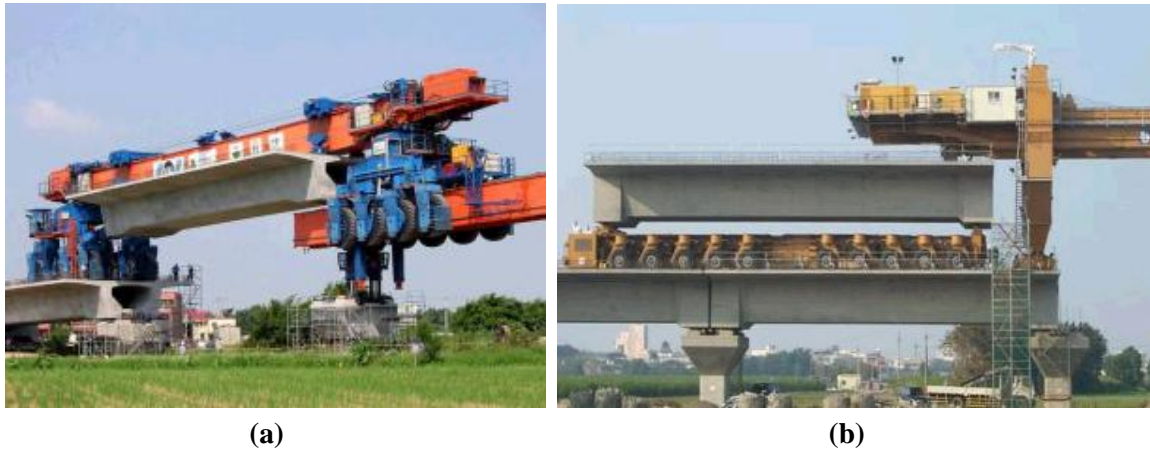
Figure 3. Full span precast erection using carriers: (a) Taiwan High Speed Contract C210-2015 by VSL; (b) Taiwan High Speed Contract C260-270 by Continental Engineering Corp
