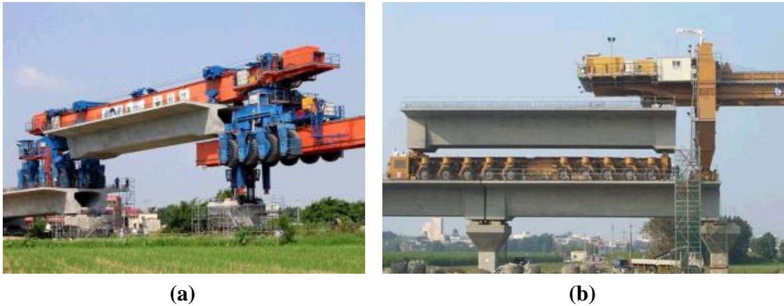
Figura 3. Plataformas de transporte: (a) Taiwan High Speed Contract C210-2015 by VSL; (b) Taiwan High Speed Contract C260-270 by Continental Engineering Corp.
