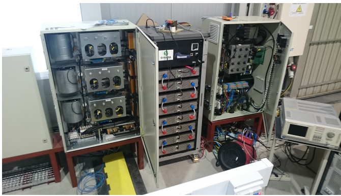
Fig. 13. Main power converters of the microgrid lab used for the system testing.
