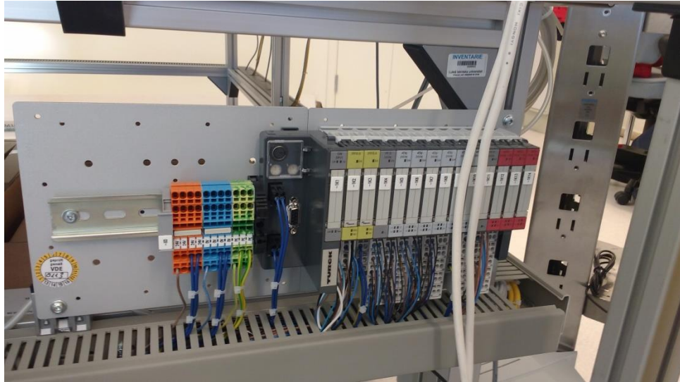
Figure 4. PLC spot with I/O and communication controller
