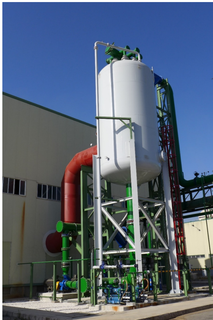
11 12 Figure 3. Steam absorber detail at the “Vetejar” biomass power plant.
