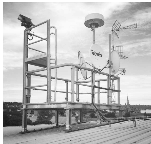
Fig. 2. Antennas on the balcony at the University of Oviedo.
