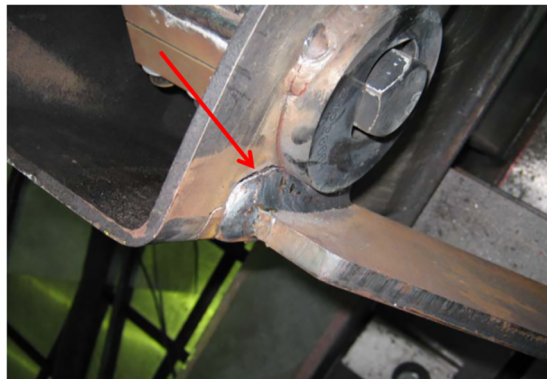
Fig. 43. Detail of the crack in one of the axle bracing supports after a 3-T load fatigue test.
