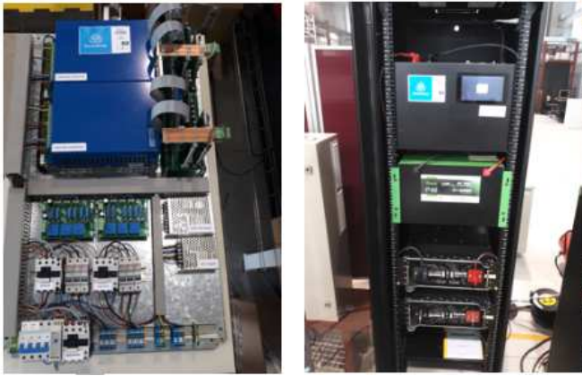
(c) Left: Setup of the converter and control for the system. Right: energy storage subsystem (up: BMS. center: Li-Ion Battery. down: Supercapacitor Modules).
