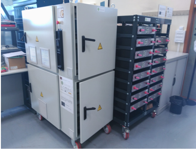
Figure 1.4: Power converter (left) with the batteries (right).
