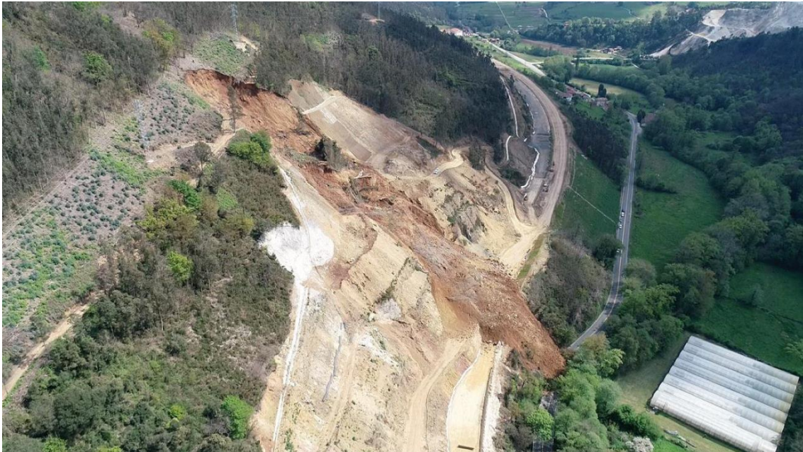
Figure 3. Complex movement developed in the A-66 highway works in Cornellada town (Asturias) on April 16, 2021. Its triggering was linked to rainfall and anthropic activities. Photo taken by the La Nueva España newspaper.
