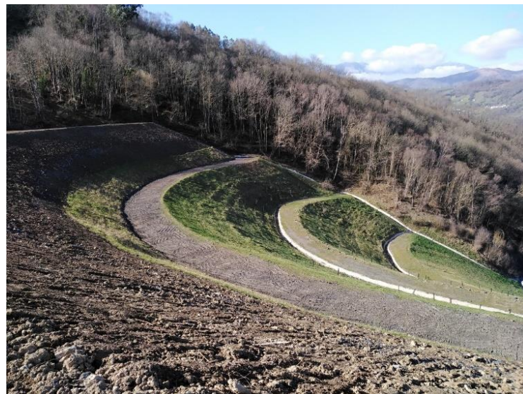
Figure 1. Sector two of the waste heaps area of the Figaredo mine is being restored.
