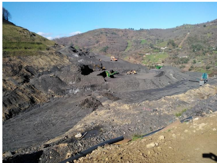
Figure 2. Sector four of the waste heaps area of the Figaredo mine is being re-exploited for coal recovery.
